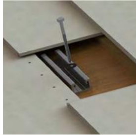
2. Insert the lag bolt through the Tile Strut and apply compatible sealant.
